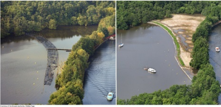
Figure 4: Salhouse Spit (i) eroded area showing line of geotextile bags and (ii) after placement of dredged sediment
